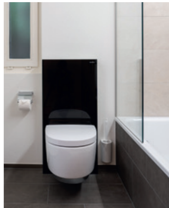
AFTER Installation situation with Geberit Monolith
