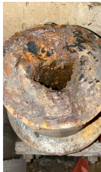
Congealed waste had reduced the bore of the 4-inch soil stacks to just over an inch in some places
