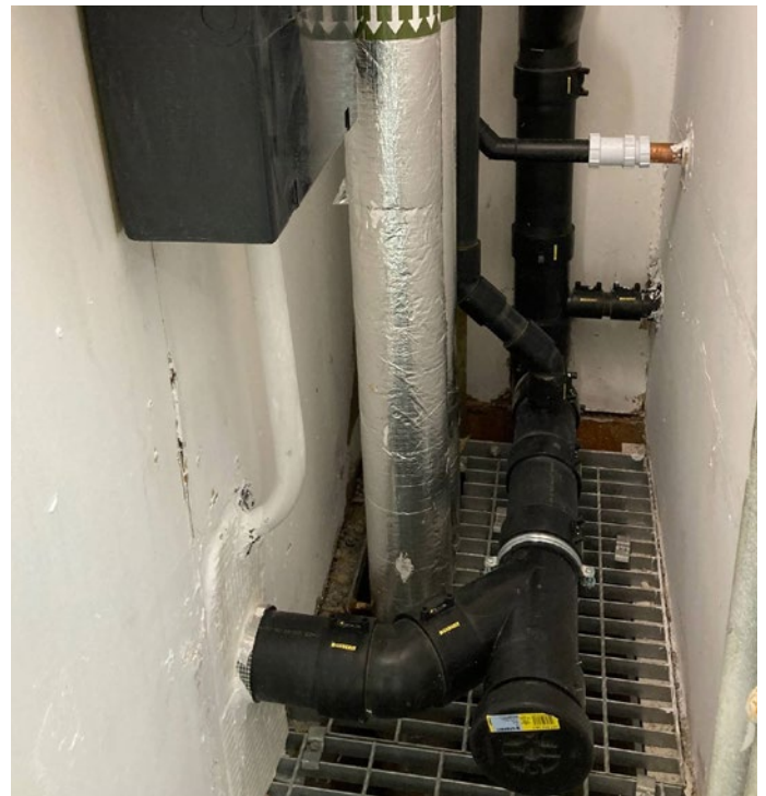
A cleaning access point at the bottom of a new Geberit HDPE soil stack
