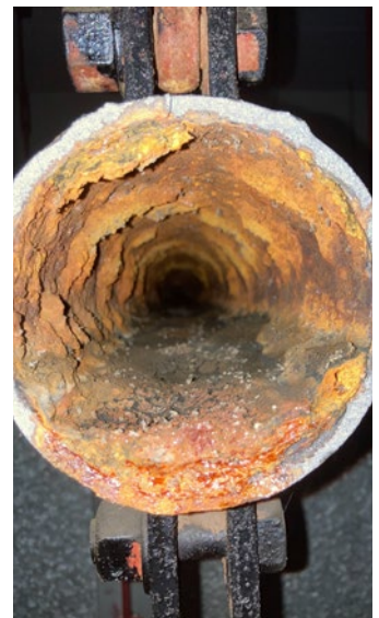
A cutaway image showing internal narrowing at a horizontal section at the bottom of a soil stack
