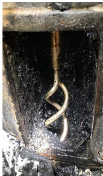
A worm screw pictured through an open cleaning eye as staff attempt to clear a blockage
